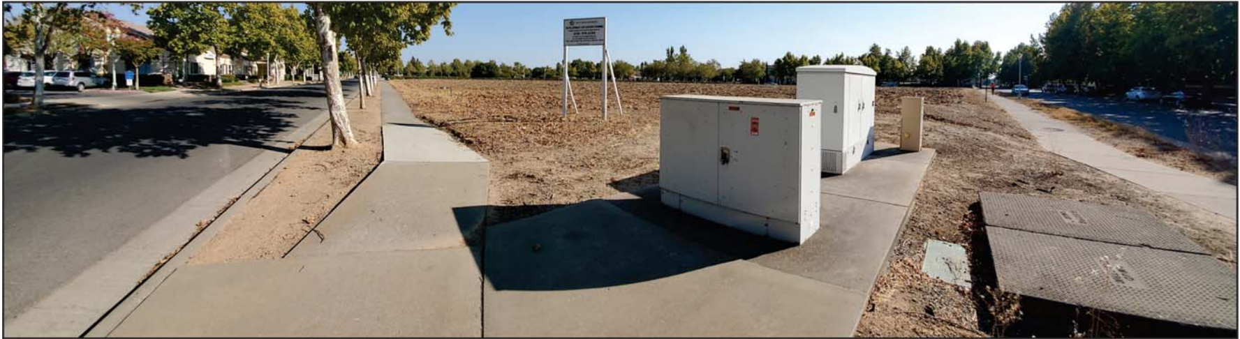
Photo 1: View of the subject property from the northwest corner. Transformer boxes on a concrete pad were observed.
